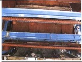
Boiler Panel 鍋爐板
